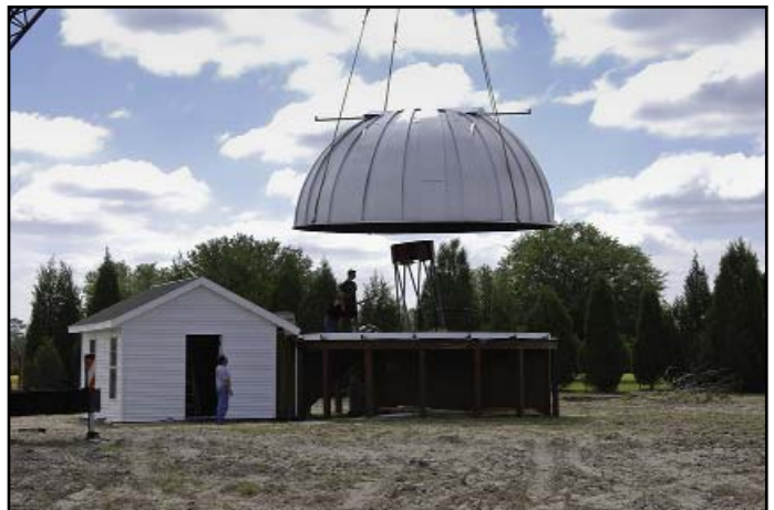
The aluminum dome is so light that the crane could have lifted many of them at once.
