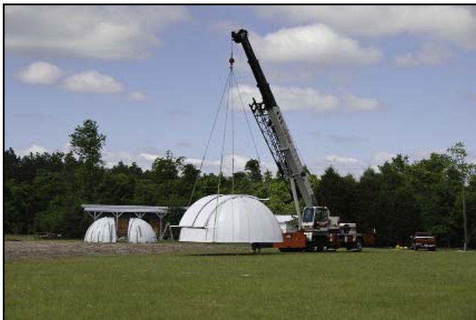
Novak watching the crane drive the dome over to the new home. The 16' dome can be seen in two pieces in the background
